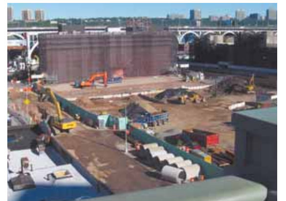
View of Manhattanville construction from the elevated subway station at 125th Street
